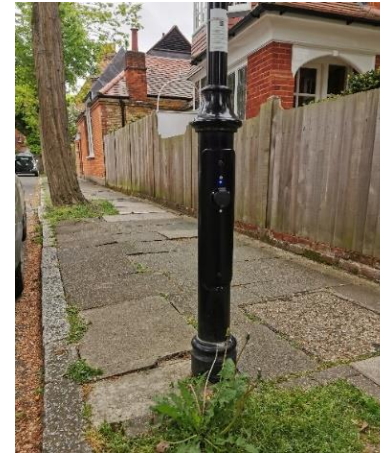
Fig 9-5: Lamp post chargers (slow) must only be incorporated into lamps when they are placed on the edge of the pavement and carriageway to avoid trailing cables across the pavement (Credit - Create Streets)
